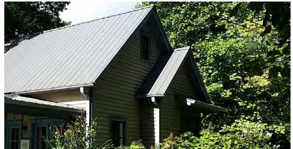
Below, the inappropriate use of a nested gable that is bumped out less than four feet, likely only to provide visual interest to the facade.
