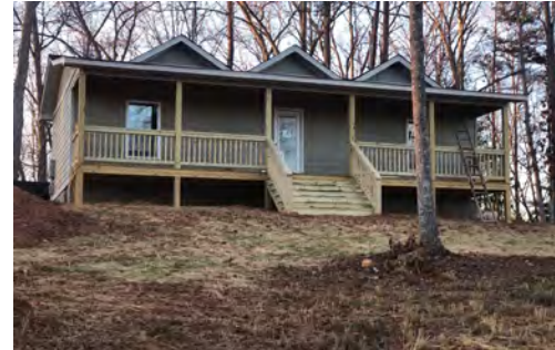
NO - Porch is not enclosed and is unpainted
